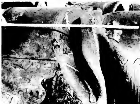
Photo 5. Granada trunk line. One of the more severely damaged welded slip joints. Los Angeles Department of Water and Power photo.
